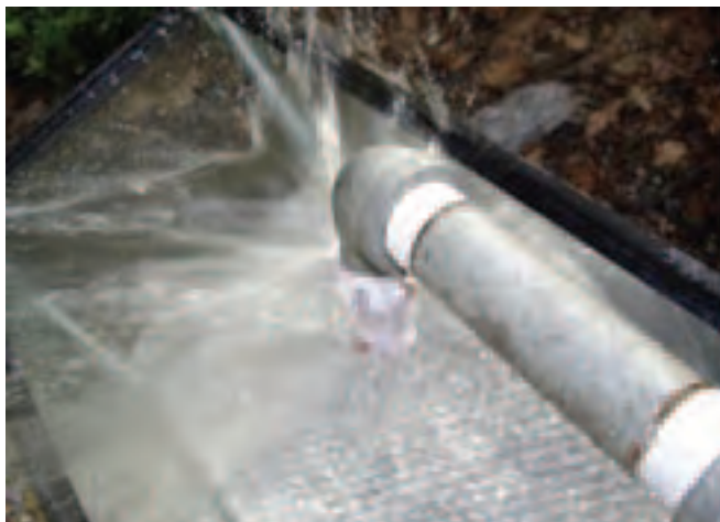
Figure 6 - Some plastic bags that exhibited shrinkage were found to obstruct sprinkler spray patterns
