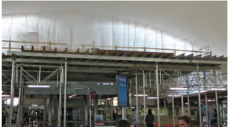
Major remodel and still no sprinklers
