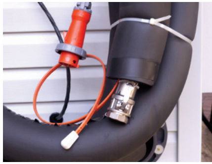
Closeup of Water Hose
