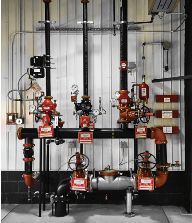
Fire sprinkler riser manifold with backflow preventer.
