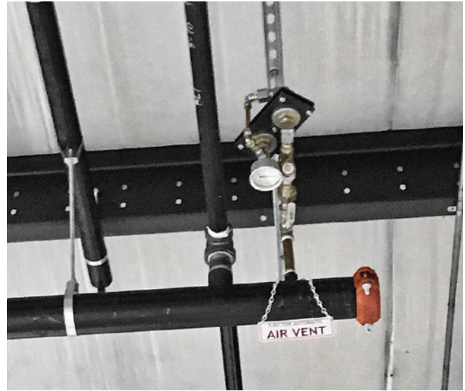
Air Venting and System Piping in the Apparatus Bay.
