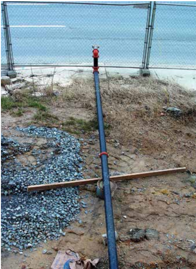
Figure 2. Temporary standpipe connections should be clearly marked and remain unobstructed so the fire department can find and use them quickly.
