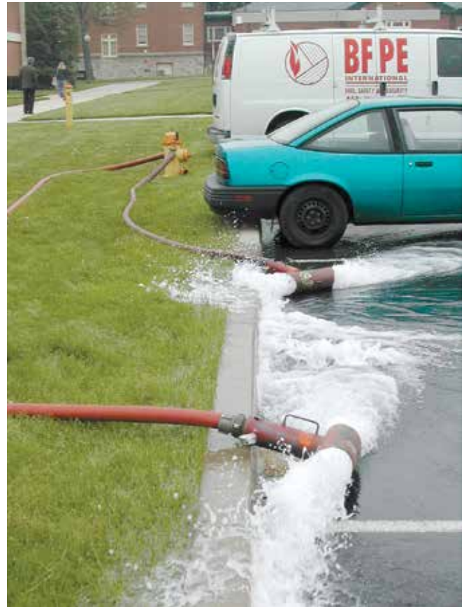
Figure 1. Flow test results used for sprinkler calculations can be shared with the local fire services so they know what to expect in case of a fire during construction. (All photos by the author).
