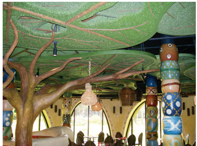
Then, there is what our group refers to as the car wash, on a water ride, with an opening where a fire wall was not practical or achievable. The tradeoff was the installation of a deluge system to protect the opening.
