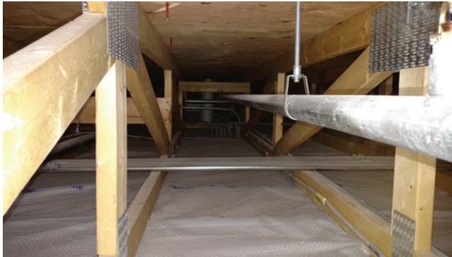
Attic with sprinklers and without draftstopping
