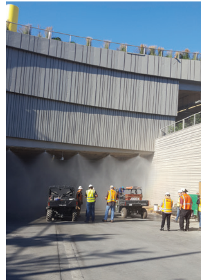
Testing of the deluge system in the new Washington State SR 99 Tunnel took two months to complete, and drew a lot of interest from the media and the public.
