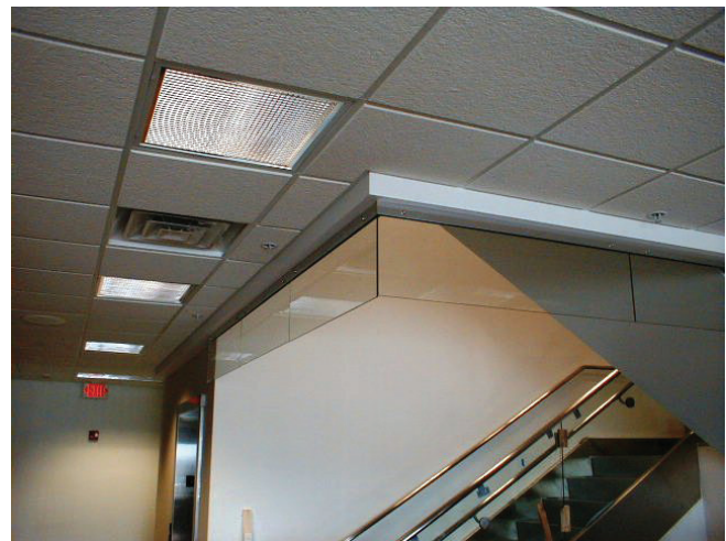
Stair with draft curtain and closely spaced sprinklers
