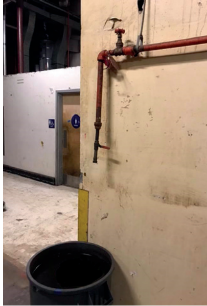
Inspector's test valve not piped to suitable location
