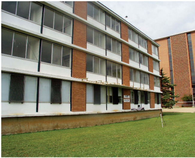
Figure 6 - Photograph of the outside of the northwest wing of the dormitory building looking southwest
