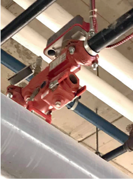
Floor control assembly No drain connected
