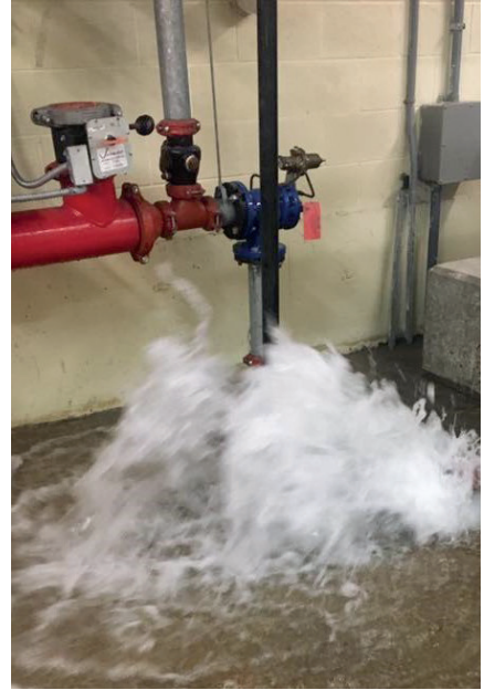
Pressure relief valve dumping in a fire pump room
