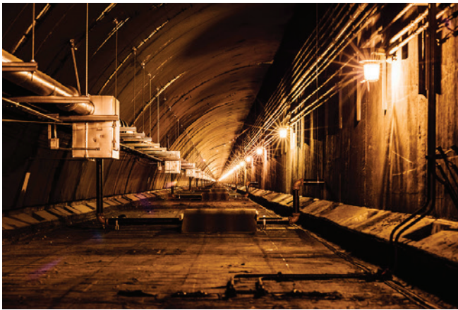
Eisenhower Tunnel - Supply Plenum Looking East
