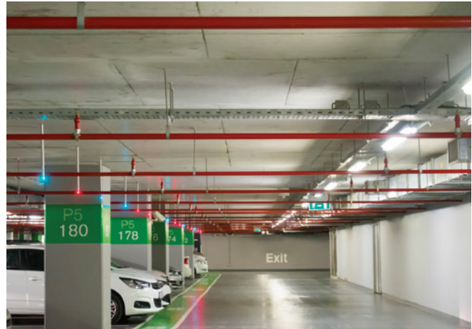
Small, temperate parking garages are considered partially conditioned spaces that can use listed antifreeze.
