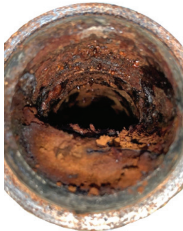
Corrosion performance of listed antifreeze is especially important to consider for metallic piping systems.
