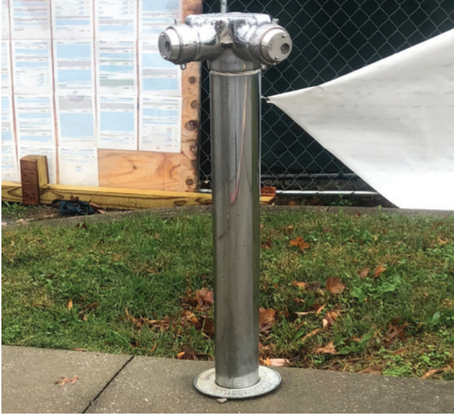
Standalone Siamese Fire Department Connection.
