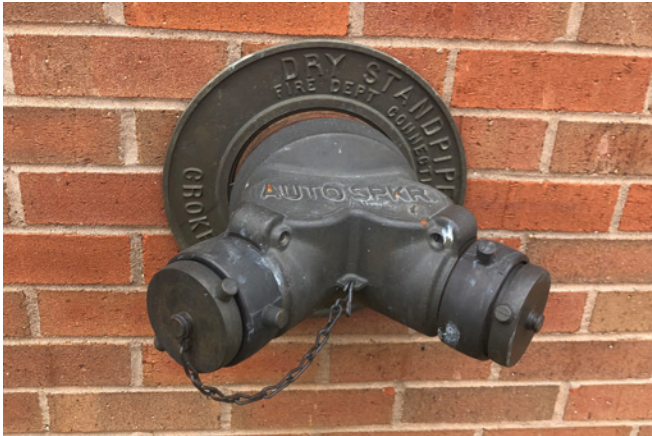
Wall mounted Siamese Fire Department Connection.
