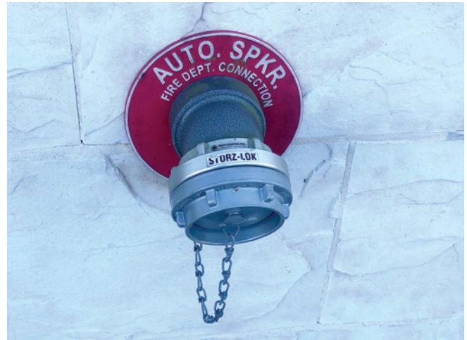
Storz Fire Department Connection.
