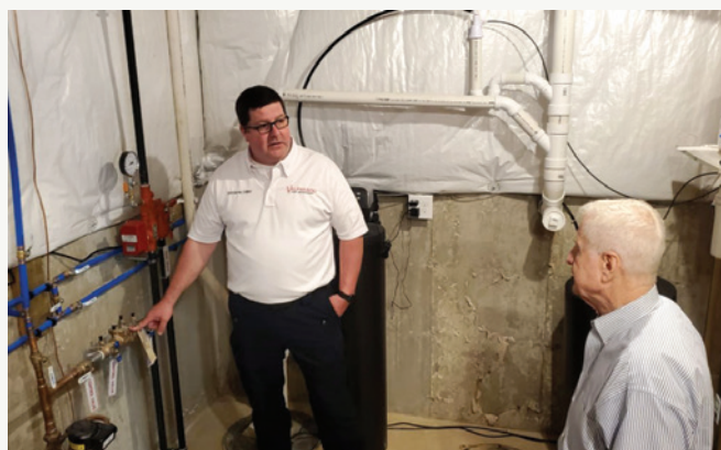
Valparaiso Division Chief Tim Stites shows Indiana State Senator Ed Charbonneau components of the home sprinkler system.
