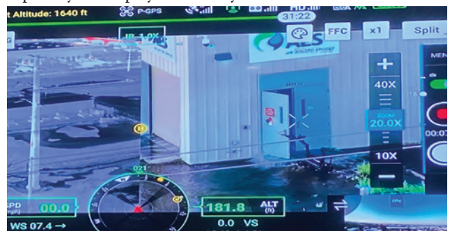
UAV screen capture of a law enforcement robot opening the door to the building housing a 10 MW/Hr. ESS.
