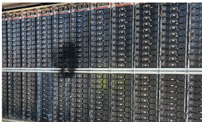
The automatic sprinkler in the module protected the ESS system from thermal runaway cascading to the adjacent modules.
