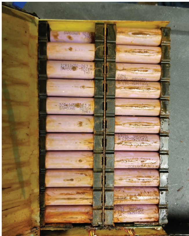
The 12" wide x 9" deep x 17" long enclosure contains 66 LiB cells & the energy storage management system.
