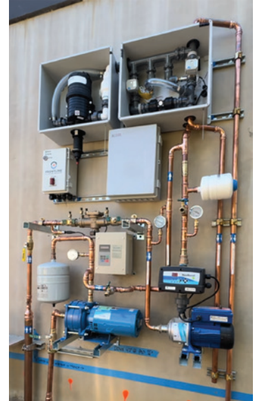
Frontline System installed by Jason McDonough with SoCal Wildfire Defense Systems
